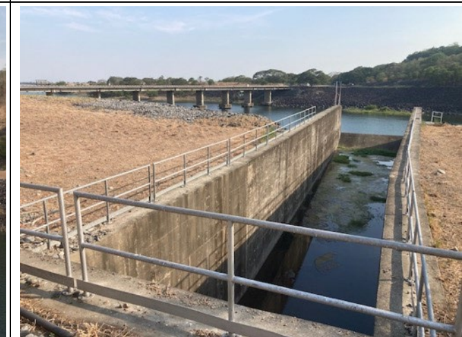
Photo 48: Low-level outlet, not used for a considerable time
