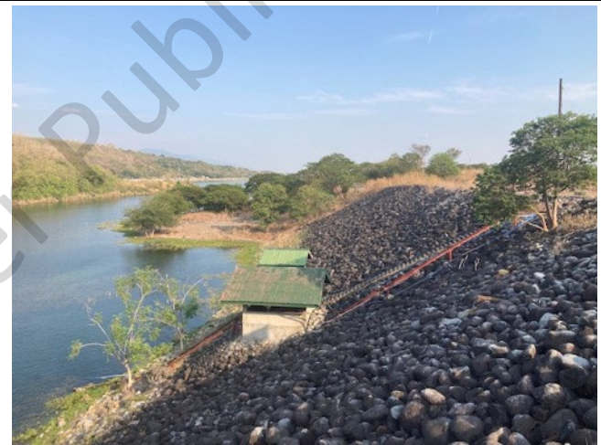
Photo 53: Pumps providing domestic water for SRPC camp and offices
