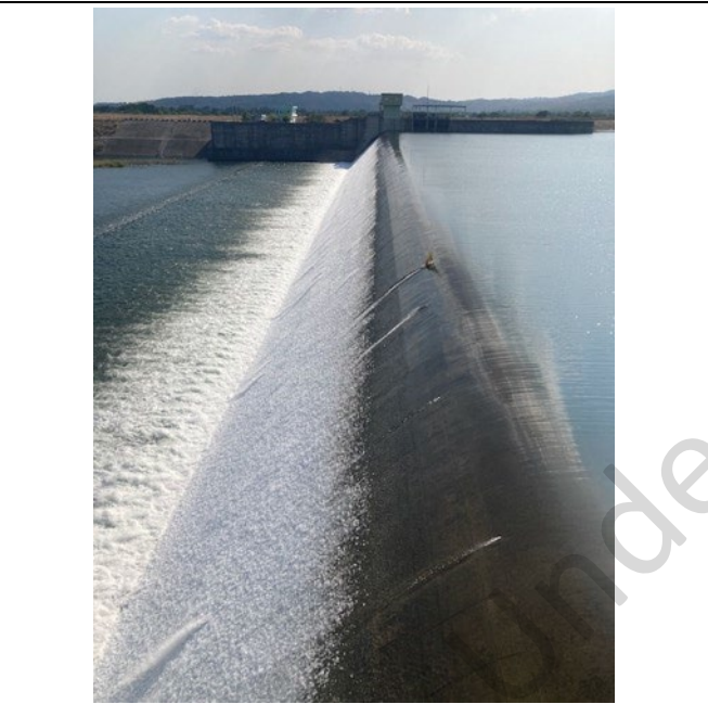
Photo 82: Weir of re-regulating pond spilling between irrigation seasons
