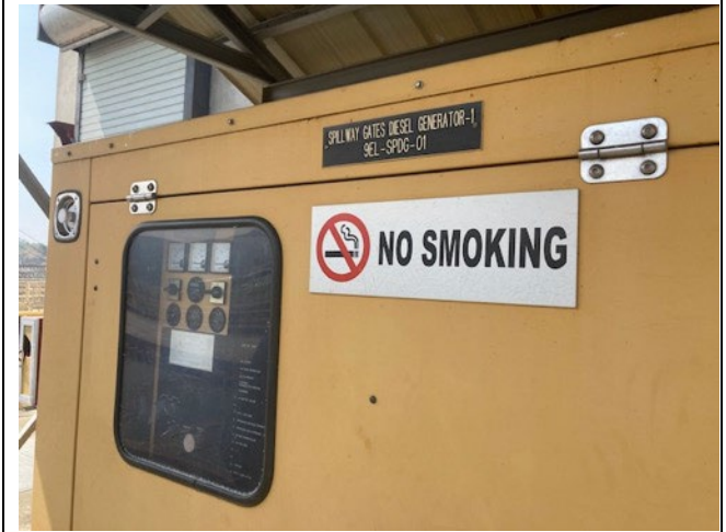
Photo 24: Spillway gates backup diesel generator
