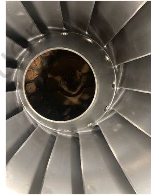
Photo 33: Turbine runner in good condition during maintenance
