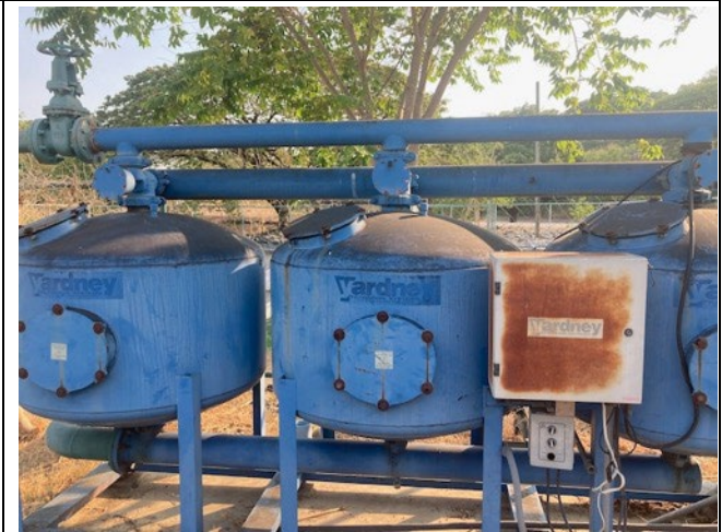
Photo 54: Water filtration for operator's village
