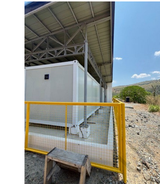
Photo 88: Chemical storage with containment
