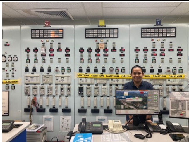
Larawan 34: Control room
