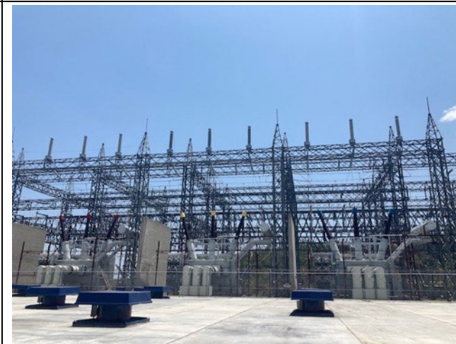
Larawan 30: Switchyard at bubong ng powerhouse
